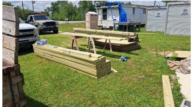
A new ADA, wheelchair accessible ramp being added to a home to accommodate owner with limited mobility.
