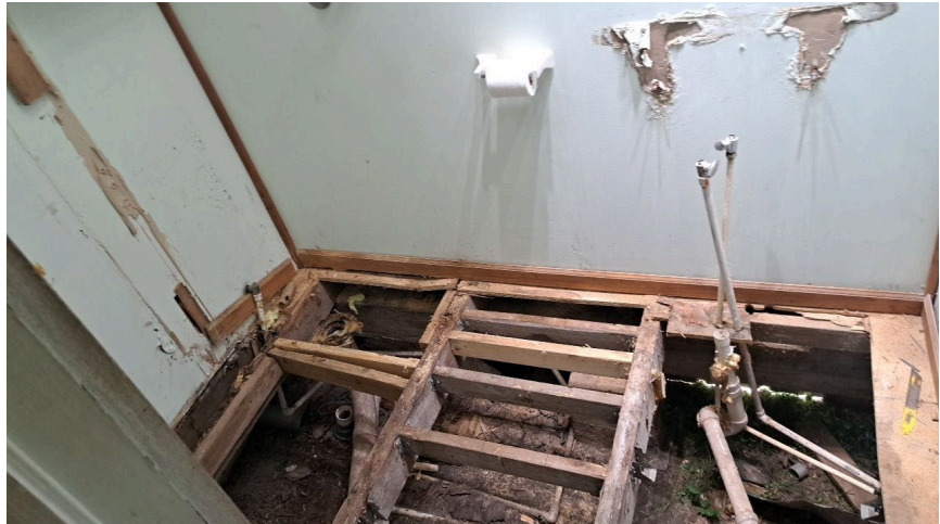
Above: Photo of rotten flooring system to be replaced with new floor system, sub floor and floor covering.
