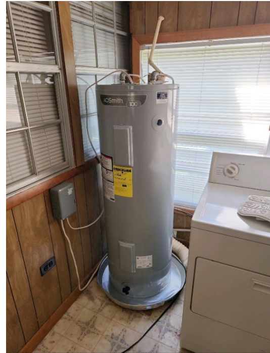
Above: A new, energy efficient hot water heater was added to a Jackson County home using SHIP program funds.
