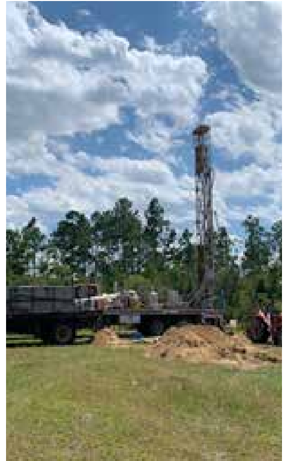
Above: Photo of new well installation to ensure safe drinking water for HHRP applicant following damage from Hurricane Michael in 2018.
