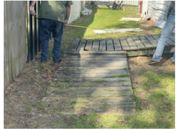
A Contractor taking measurements on a ramp for an Owner-Occupied Rehabilitation project during bid walk-through day.
