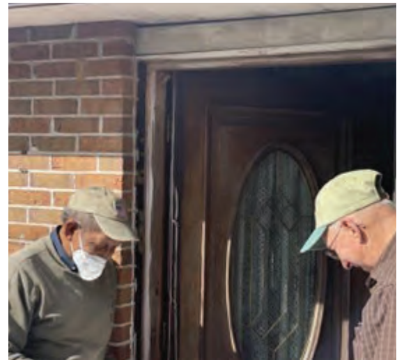
A Contractor and the Program Home Inspector together for a bid walk-through at a resident's home.
