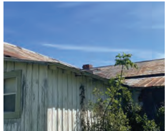
The home of an applicant, who's roof is being assessed for Owner-Occupied Rehabilitation.
